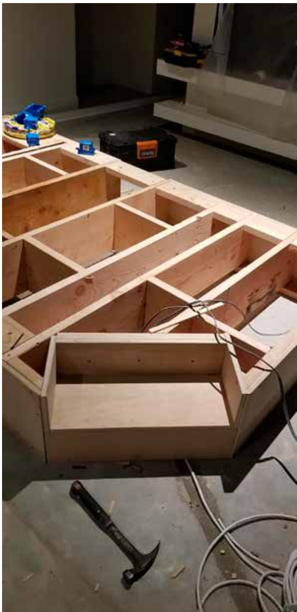
A FIRM FOUNDATION: Custom home installations are hand built from the bottom up.
